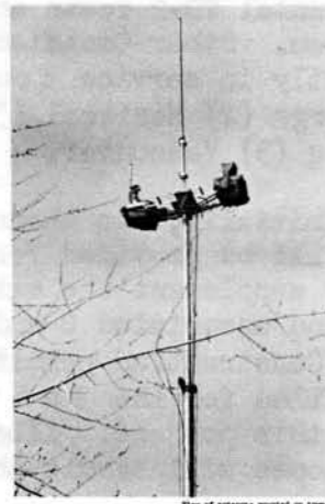
View of antenna mounted on tower.
