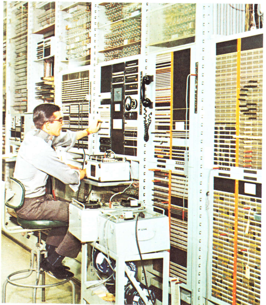
Installer testing Centrex equipment from the Master Test Frame.
